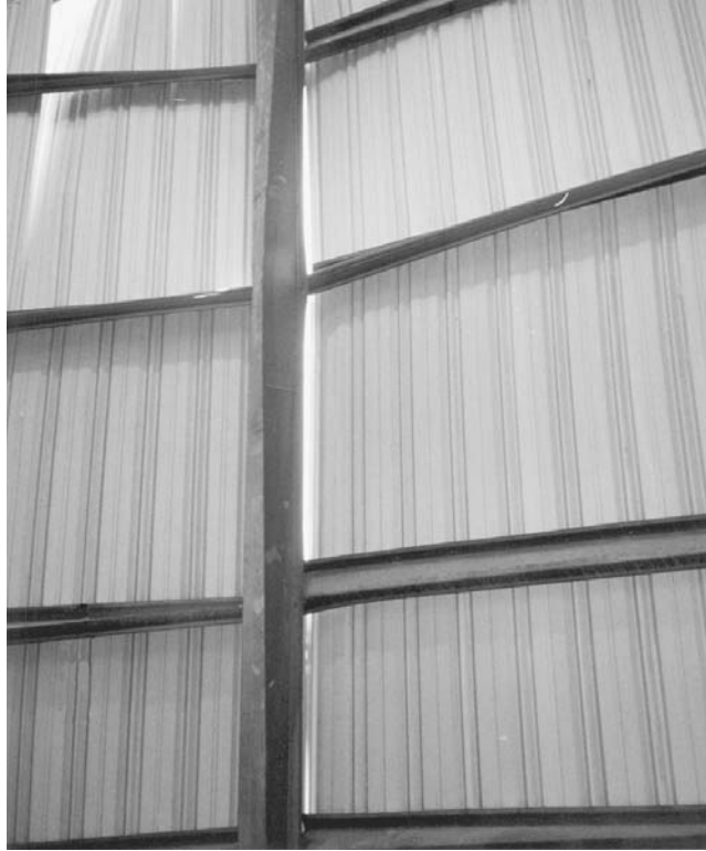
FIGURE 10.18 Buckling of laterally unbraced girts and endwall column under wind loading. (Photo: J.R. Miller & Associates.)
